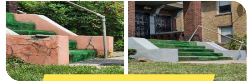
Through the AHIP program, these concrete steps were repaired for an Avondale resident.
